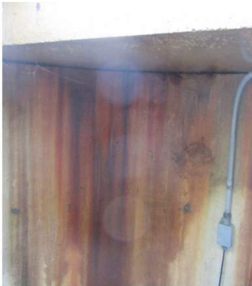
Signs of infiltration under valve chamber lid
