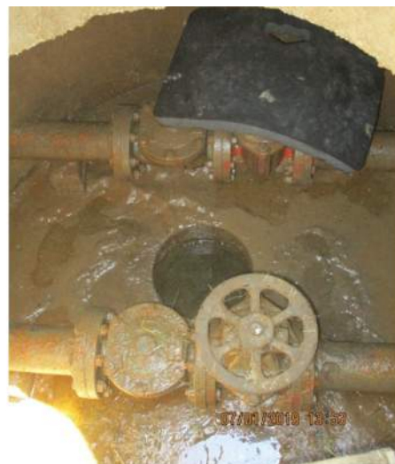
Corrosion of valves and piping, accumulation of solids in valve chamber
