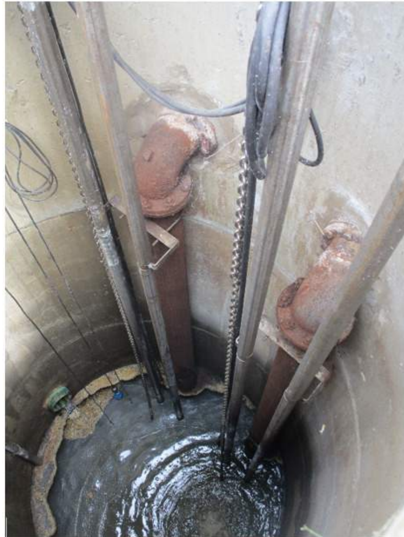
Corrosion of wet well piping, flanges grouted into wall
