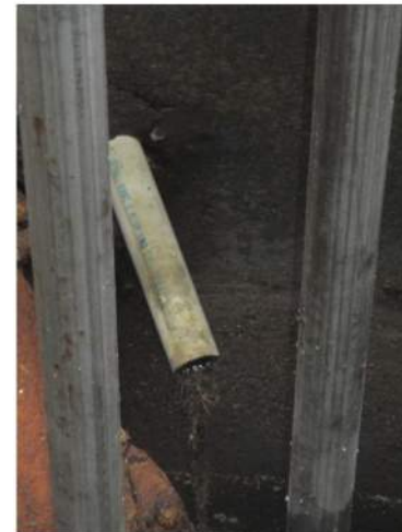
Valve chamber drain pipe partially clogged with roots
