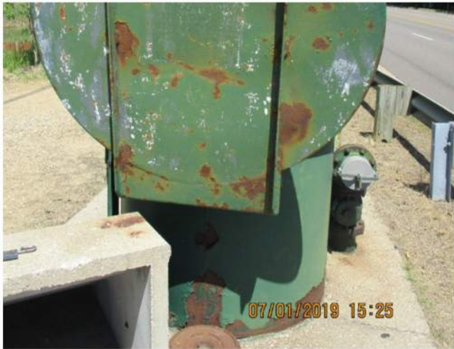
Corrosion of can exterior
