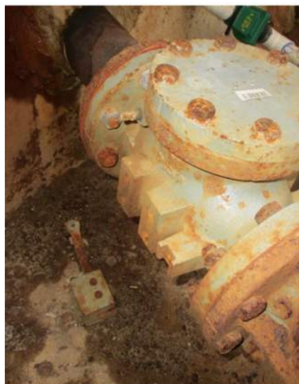
k valve lever arm, corroded valves
