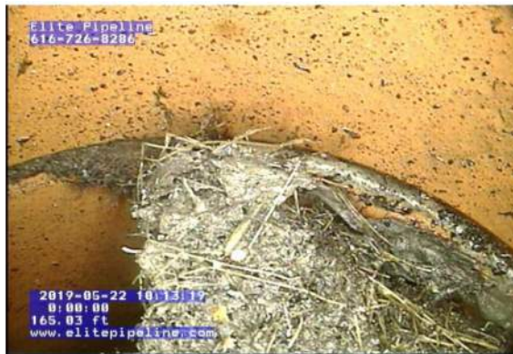
Roots (Joint) – 170' Downstream MH 05654 Drake Road
