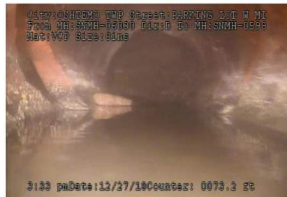
Broken Pipe – 73' Downstream MH 06030 11 th Street
