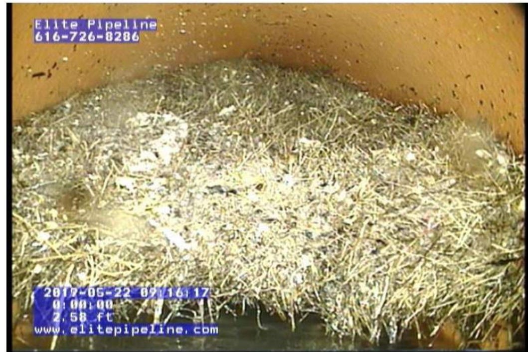
Roots (Ball Barrel) – 257' Downstream MH 05654 Drake Road
