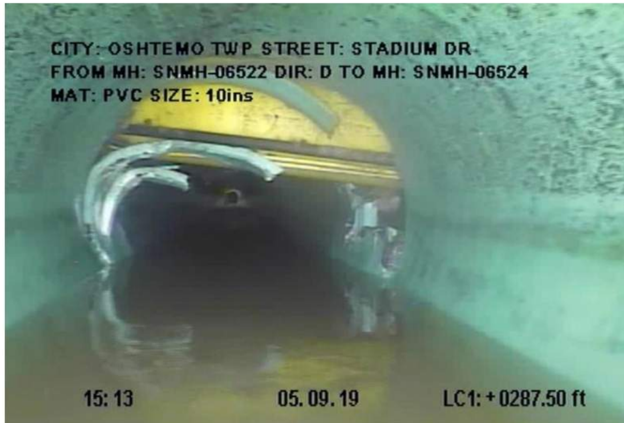
External Utility Penetration – 288' Downstream MH 06522 Stadium Drive
