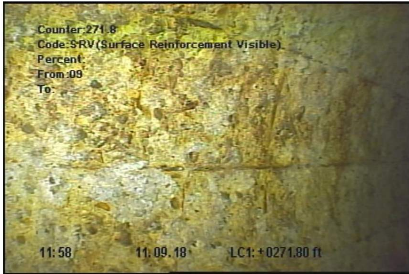
Surface Reinforcement Visible – 13' Downstream MH 05990 Antiqua Circle
