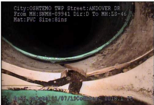
Broken Pipe – 18' Downstream MH 09941 Andover Drive
