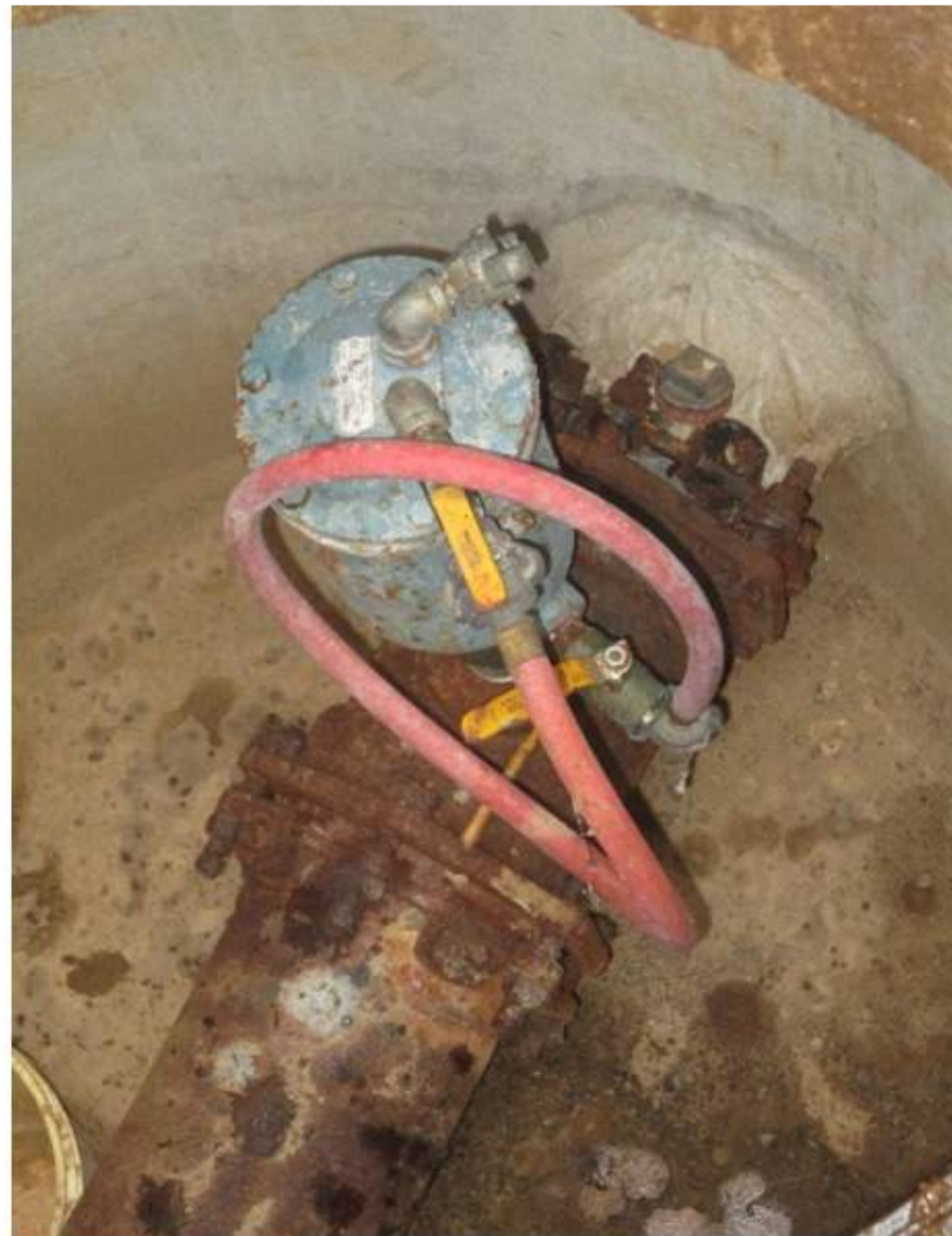
Corrosion of air release structure piping, valve in poor condition
