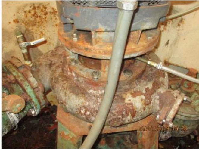
Corrosion of Pump No. 2
