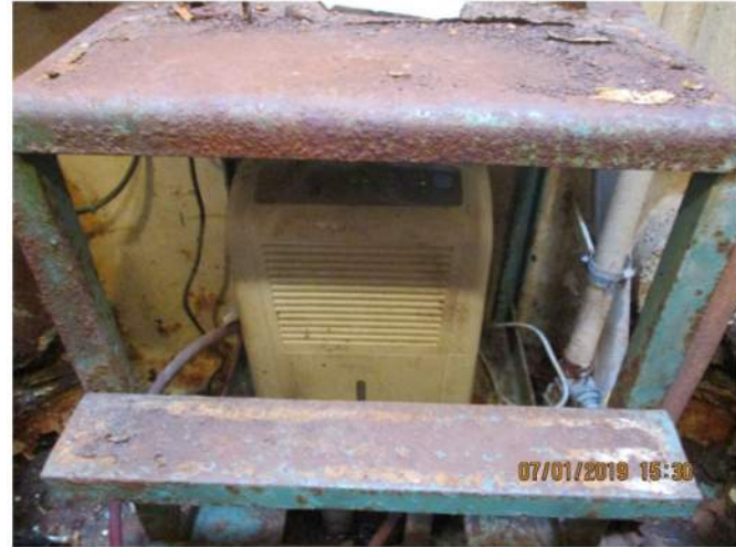
Dehumidifier in poor condition
