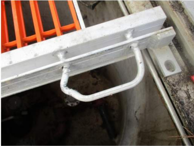
Broken valve chamber safety grate handle
