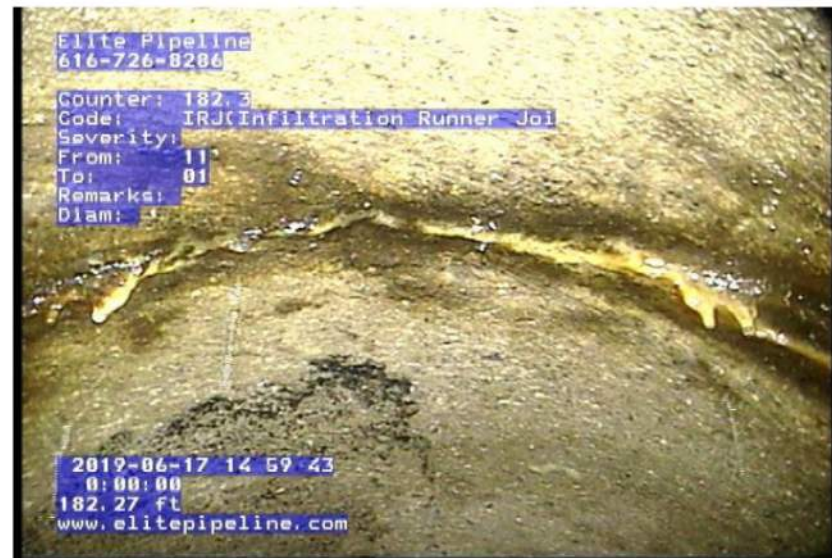
Infiltration Runner – 272' Downstream MH 05718 W KL Avenue
