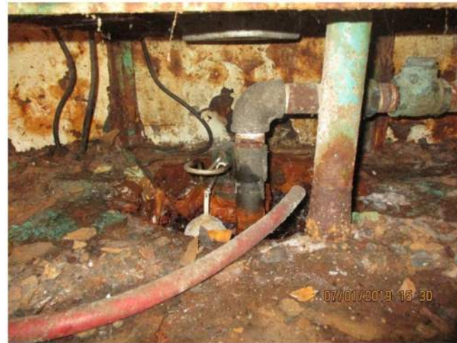
Corrosion of can floor, sump pump, and piping
