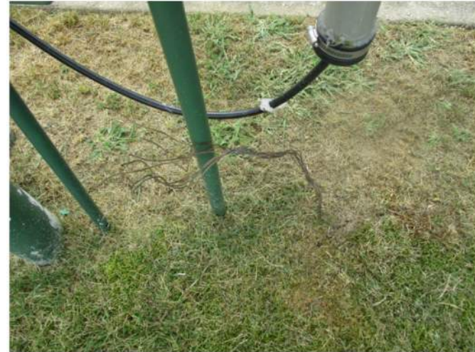
Grounding electrode not connected to control panel
