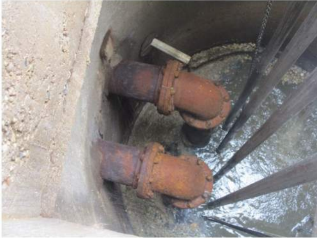
Corrosion of wet well piping
