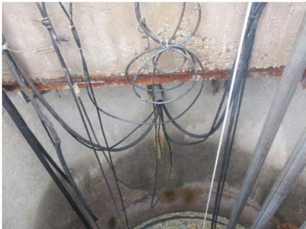
Intrinsically safe instrumentation cables in same conduit as pump cables
