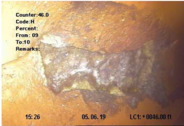
Broken Pipe – 295' Downstream MH 06208 9 th Street
